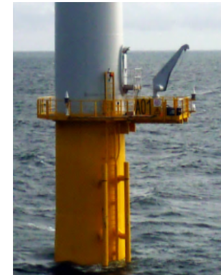
Transition Piece Including boat landing for service vessels
